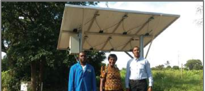
D&S TZ under GM Ben Munyao has been active with a large number of solar installations, one such being for a farm in the Dodoma region. Solar powered pumping solutions are ideal in Tanzania where remote locations are not connected to the grid. Pictured is happy client Mercy Mtei and Ibrahim Ikisungwe with D&S staffer Kheri Haule.
