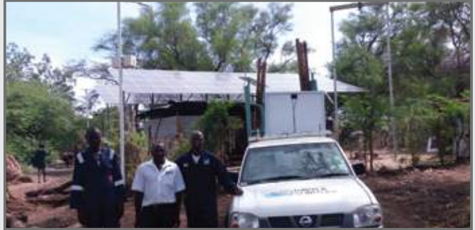
Pictured is James Ekhai and Dickson Nyakenyanya from Norwegian Refugee Council (NRC), one of the NGO's partnering with UNHCR, and D&S Technician Michael Kioge during installation of solar boreholes at the Kakuma Refugee Camp.
