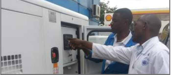
D&S Uganda under Commercial Director Simon Batte is carrying out extensive off-grid power supply projects for the National Water and Sewerage Corporation as they expand their countrywide water distribution network. Pictured is a Dayliff Perkins genset being installed at Kanyanya substation by Technician James Sitati.
