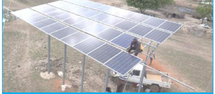
D&S Juba, under Country Manager George Kinyanjui, operates under the harshest of conditions but has never the less successfully completed 7No large solar powered borehole installations in remote parts of the country. These installations will now provide water to upwards of 60,000 people affected by insecurity. Pictured is Samaritn Purse rep. at one of the sites.
