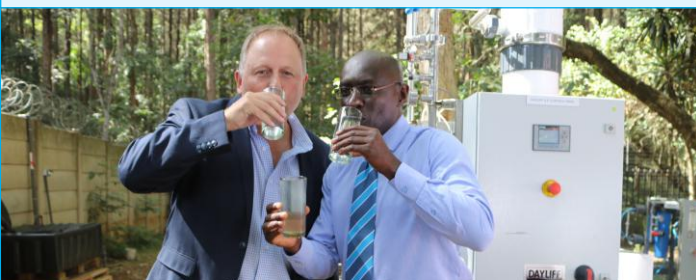
CEO David Gatende and Dow Africa Commercial Manager Don Foran are pictured as they drink the purified river water from the Dayliff DUF1 plant with Dow membranes (visible behind) as a sign of their confidence in the technology.
