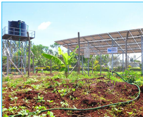
A typical solar pumping installation in Meru County, Kenya.
