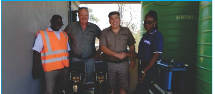
D&S Zambia under MD Jonathan Mainga has supplied and installed some booster sets for water supply at Mushingashi camp situated in Kafue National Park. Pictured are D&S staffers Chrispin Noole and Pyela Banda with Mushingashi managers Jaco Cloete and Pete Cornelius on site in the pump room.
