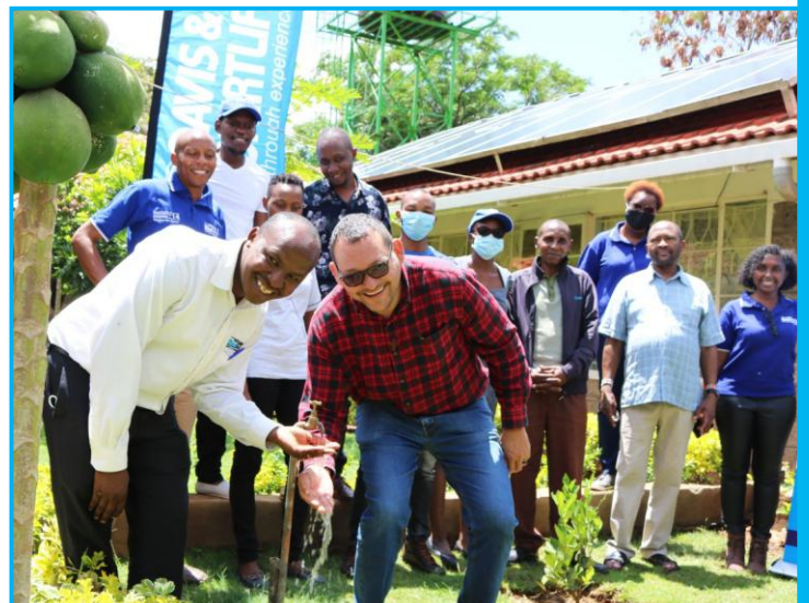
D&S HO donated and installed a solar pumping solution to Namanga Parish located at the border of Kenya and Tanzania. The team led by GM David Bolo are pictured together with members of the Parish during the hand over.
