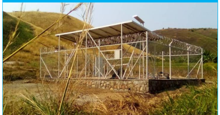
A secured solar pumping system installed by D&S DRC in Tanganyika Province in the Eastern DRC.
