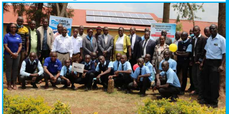
D&S HO have supplied and installed a solar pumping system at Nyakono Boys High School in Kisii. Pictured during the handover ceremony is the D&S team led by Improving Lives Coordinator Nur Riday together with students, staff and head teacher Samson Gitamo.
