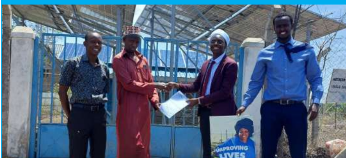
D&S Isiolo under Branch Manager Paul Muchiri have solarized a large borehole at the IWASCO showground, Isiolo town that will supply up to 20m 3 per hour to local residents. The system is powered by Dayliff equipment including a Sunverter inverter and solar panel array that will substantially enhance the sustainability of water supply to the area.
