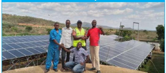
D&S Nakuru under branch manager David Ngure has supplied and installed equipment including a 75kW motor powered by a 110kW inverter to solarize Moyale county water supply. The project, which will ensure constant water supply to Moyale town, will also see the county make major savings to their electricity consumption. Pictured are key D&S and County staff at the commissioning.
