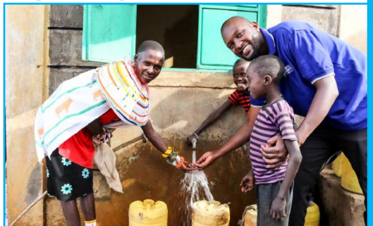
D&S Field Service Manager Lewis Njeru is pictured with members of the Suiyan community where D&S, under the Improving Lives initiative in partnership with Child Fund, supplied and installed a solar powered borehole pump which will benefit over 5,500 members of the community.
