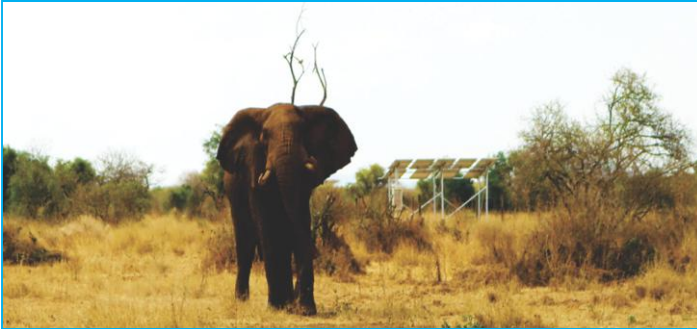
A large tusker is pictured in front the Dayliff Sunverter3 solar pumping system installed at Selenkay Conservancy.
