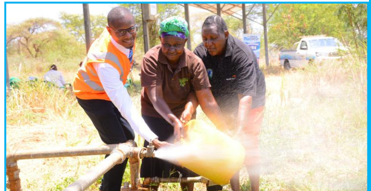
Davis & Shirliff Wote donated a Dayliff Solar borehole pumping solution to Kakuli Community that will provide constant water supply to over 5,000 community members. Pictured during the commissioning is Branch Manager Allan Ouma and community representatives.
