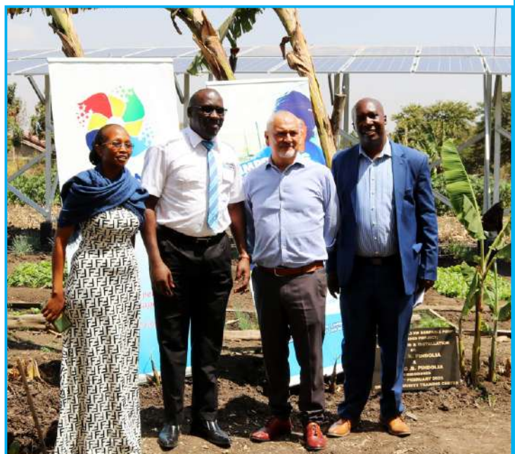
D&S under the #ImprovingLives initiative have supplied and installed a solar powered borehole pump at Don Orione community, Kandasi village. The pump will ensure constant water supply to over 400 members of the community. Pictured is GM David Bolo with Don Orione members during the handover ceremony.
