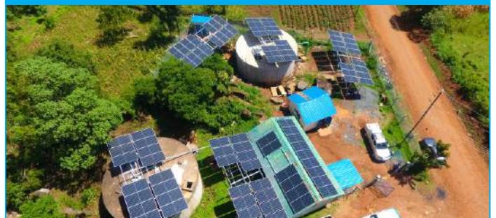
D&S Kisii under Dennis Miranyi have successfully solarized several pumpsets in Kakrao, Migori County for an engineering client. The project scope included installation of Dayliff pumps, motors, solar structures, panels and inverters. Pictured is the installation which will enable the client to reduce their energy bills significantly.
