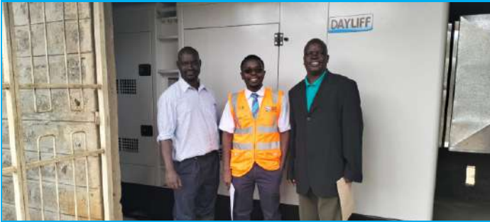
D&S Thika under Branch Manager Benson Kanyuru have supplied and installed a 250kVA genset at Juja Preparatory School Thika. The unit will provide reliable back up power during power cuts enabling students to continue with their studies. Pictured is D&S Sales Engineer Edwin Erima and school representatives Johnson Kemboi and Frederick Omondi.
