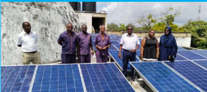
D&S Nyali under Branch Manager Adam Abdallah have supplied and installed a 55kW grid tie system at Plaza Beach Hotel. Featuring an inverter, Dayliff PV modules and accessories, the installation is projected to reduce the resort's power bills by over 50%. Pictured at the site after a successful installation is D&S Engineer Misky Mohamed and technician Raymond Kuttoh with staff from the hotel.
